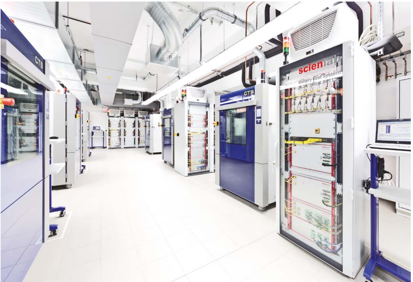
Scienlab test bench for characterization and development of battery cells and modules
